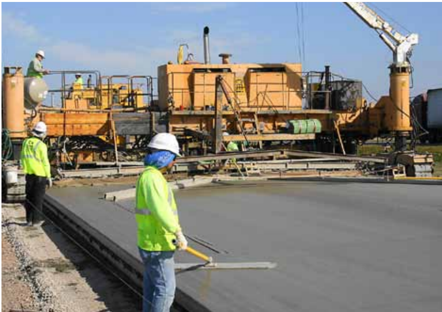
(Picture 12 – In 2009, Knife River used more than 70,000 tons of fly ash as a replacement for Portland cement during the company's production of nearly 3 million cubic yards of ready-mix concrete.)
