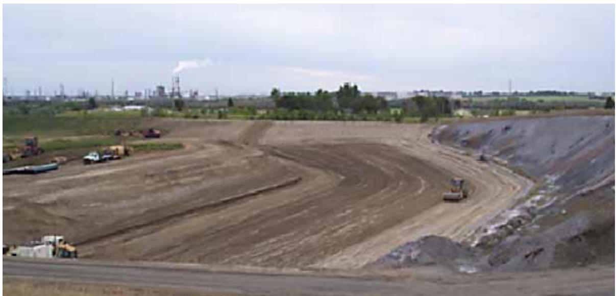
(Picture 2 – Construction crews excavating Slot 7 of the R.M. Heskett Station Active Ash Landfill, prior to liner installation. Ash in Slot 6 can be seen to the right.)
