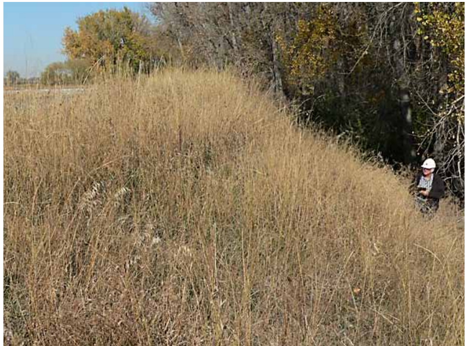
(Picture 7 – Lewis & Clark Station employee conducting an inspection of the Bottom Ash Pond embankment.)
