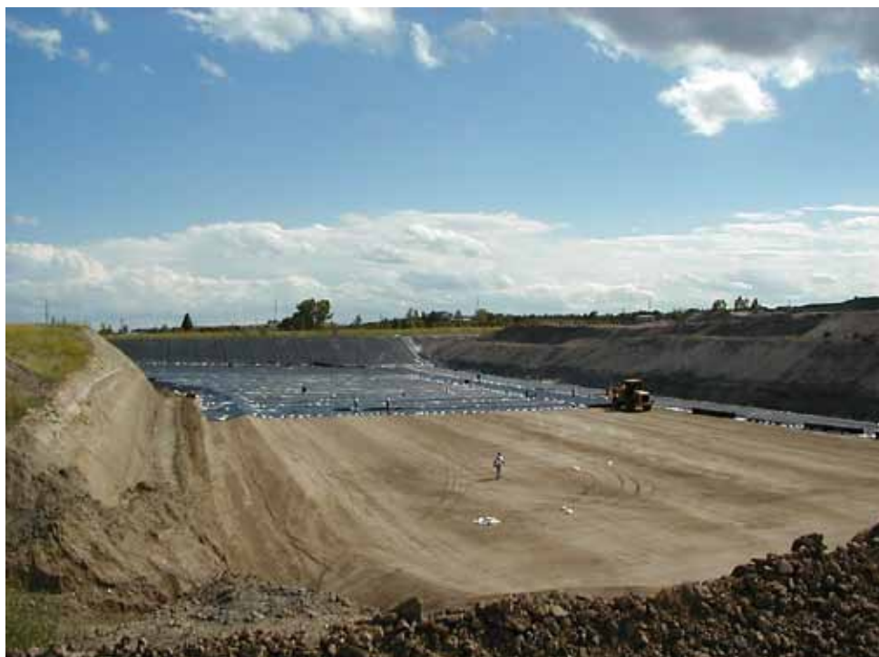
(Picture 3 – Construction crews installing the HDPE geomembrane liner on top of the engineered clay liner of Slot 7 at R.M. Heskett Station’s Active Ash Landfill.)
