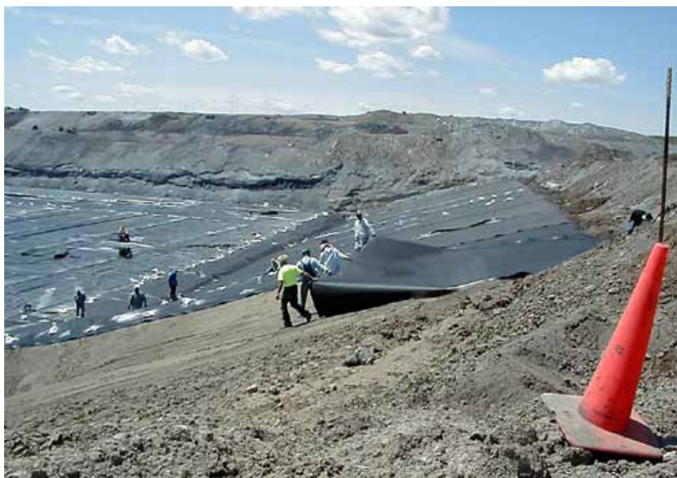
(Picture 4 - Construction crew pulling down one of the last sections of HDPE geomembrane liner during the construction of Slot 7 at R.M. Heskett Station’s Active Ash Landfill.)
